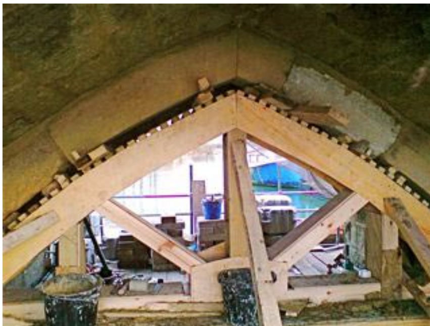
The formwork was erected off permanent scaffolding once the status of the resident bat population had been assessed.
